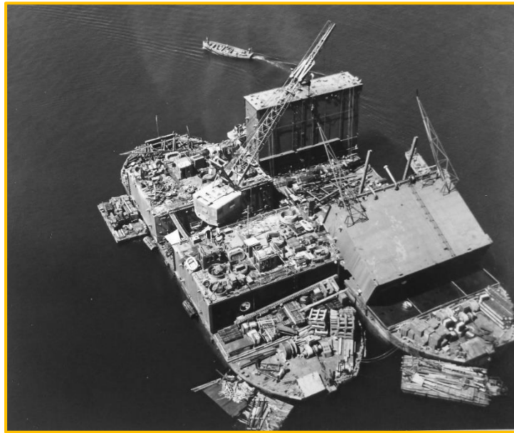
Whirly crane (Section C or D) assisting raising of the wing walls
